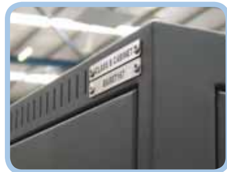
Nameplate with rack serial number
